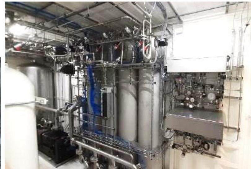
PSA Containerized System
